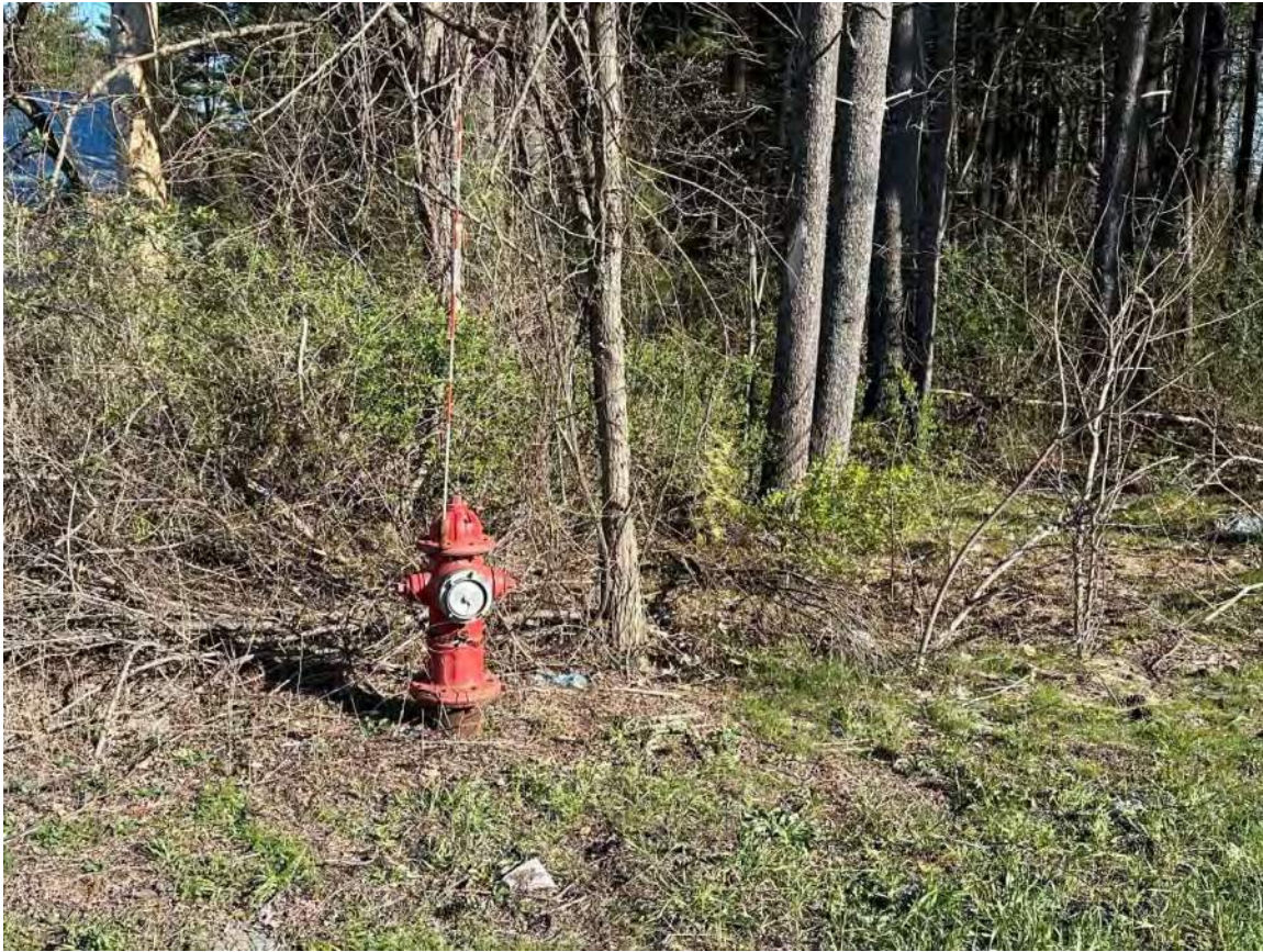
Photo 13. View of fire hydrant along the north side of US Route 9, facing northwest.
