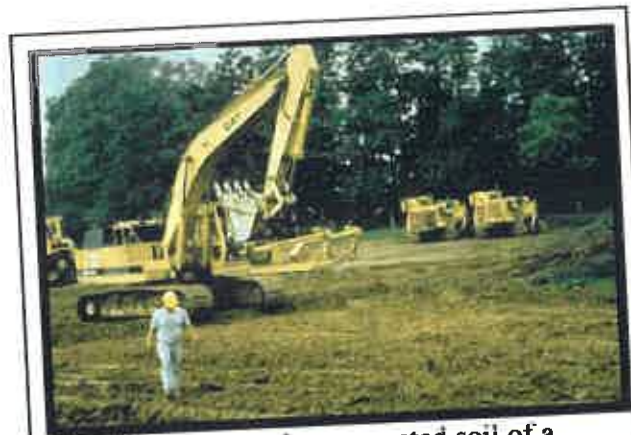
Fig. 14. The severely compacted soil of a temporary construction yard used daily by heavy equipment for four months; shown before deep ripping, topsoil replacement, and decompaction.
